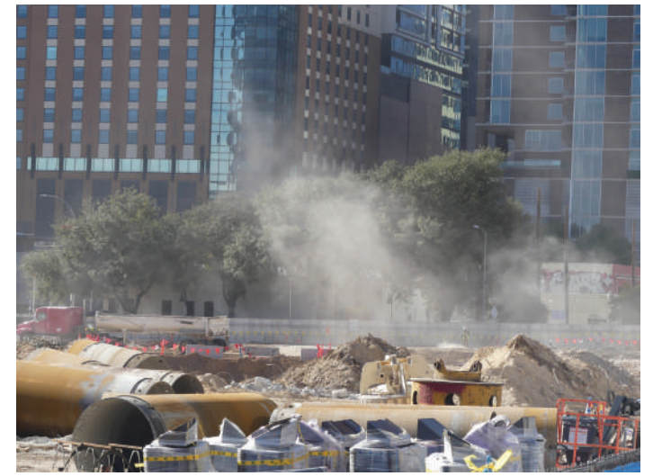
GOING UP IN DUST The early phases of the new convention center's construction continue. Currently, the site is a massive hole that accommodate its foundation. photo by Ellington Tough
